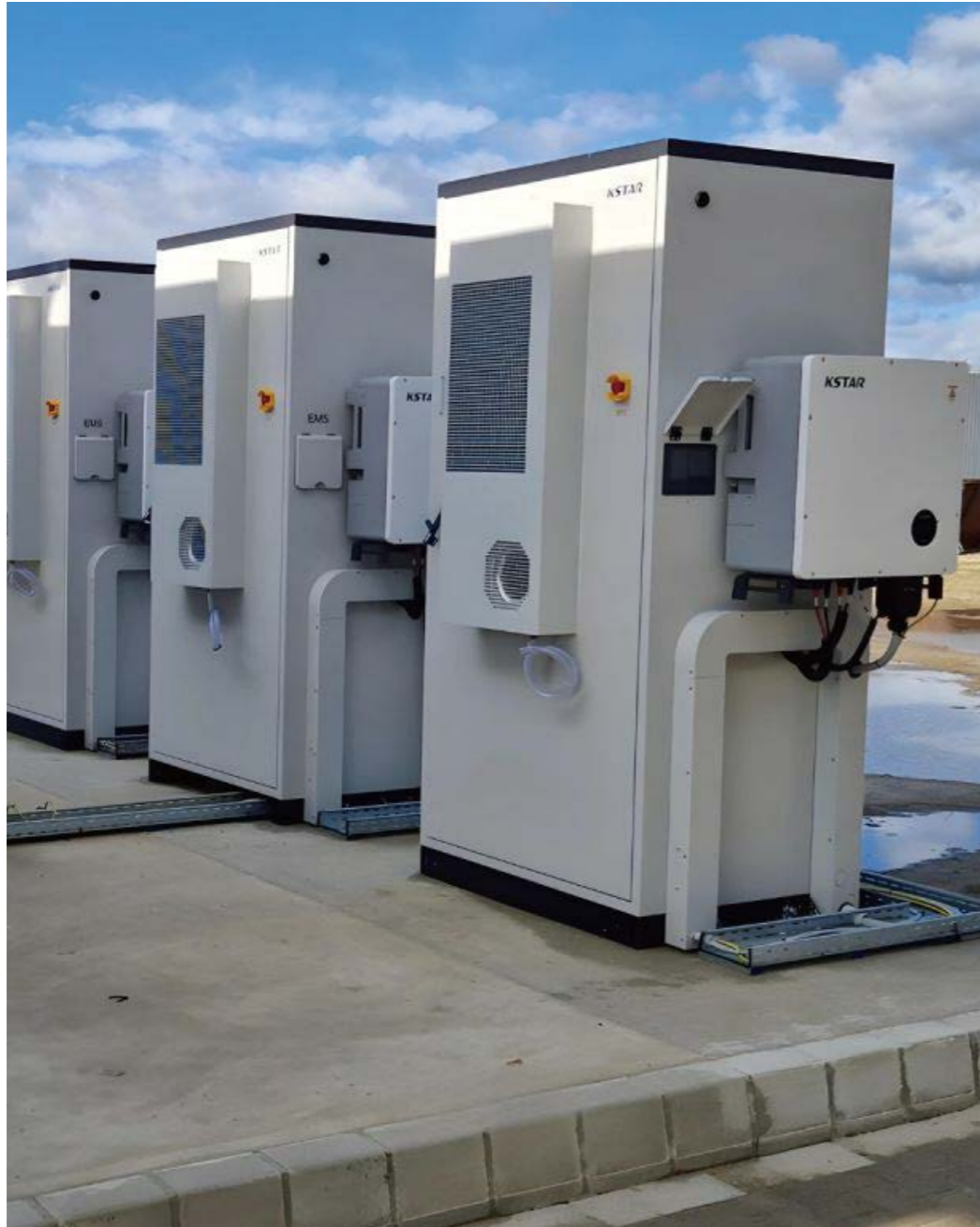
02 C&I ESS Project in Hungary
