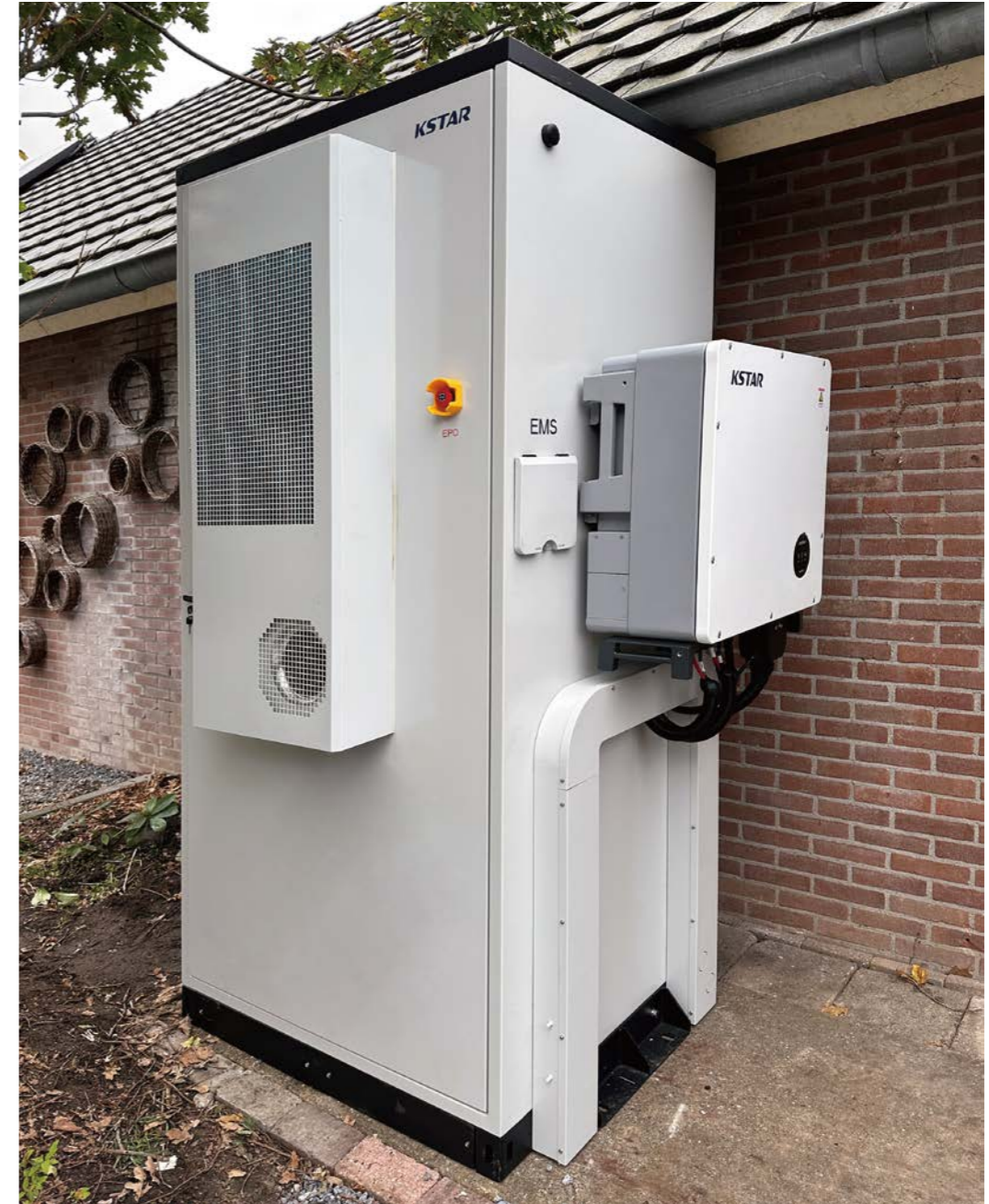
03 C&I ESS Project in the Netherlands
